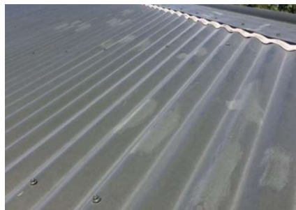
Example of excessive use of touch-up paint
