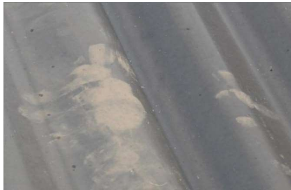
Permanent hand marking on pre-painted steel caused by contact with sunscreen
